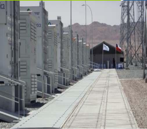
Battery Farm in Substation
