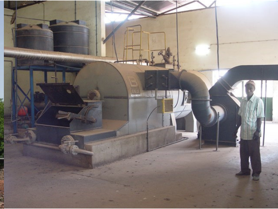
Figure 24: SICAJU biomass boiler
