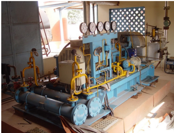
Figure 21: SAFIM steam turbine / alternator
