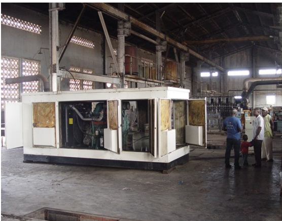
Figure 35: 450 kVA diesel generator at Bafata
