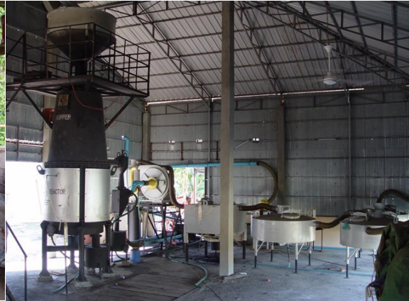
Figure 4: 200 kW rice husk gasifier in Cambodia
