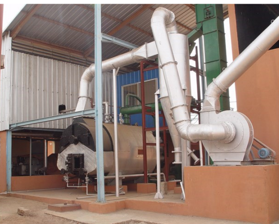
Figure 20: SAFIM biomass boiler
